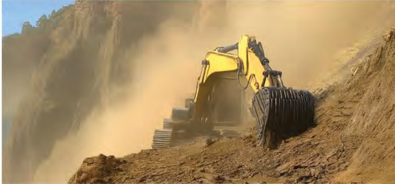
Hazardous Zone Operations
